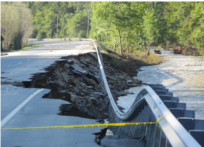
Vermont’s major East-West highway, US 4, was damaged in multiple places between Rutland and Quechee during Tropical Storm Irene, cutting off cross-state traffic. Credit: TRORC.
